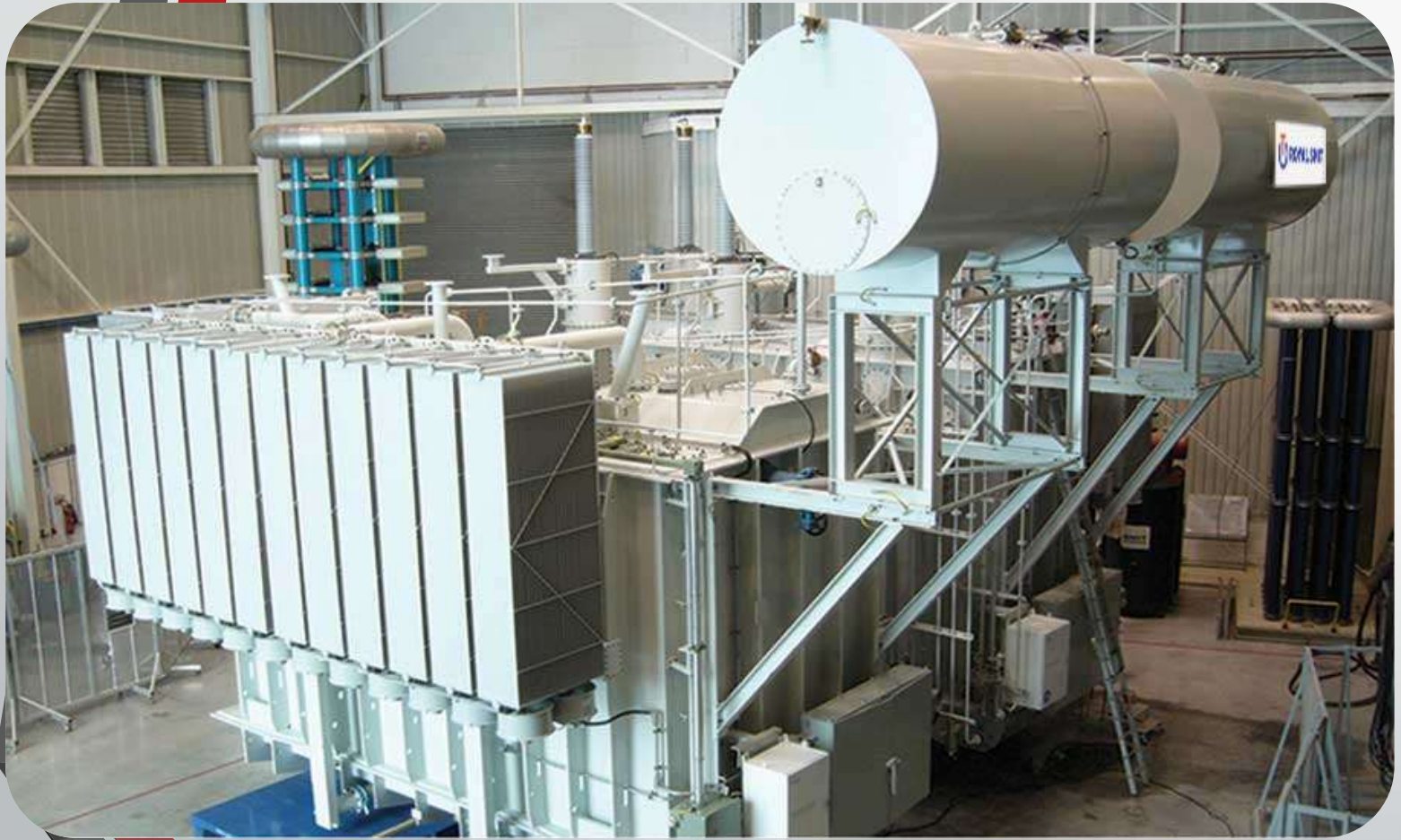
700 MVA, 240kV , \pm 30^\circ in \pm 16 steps PST
